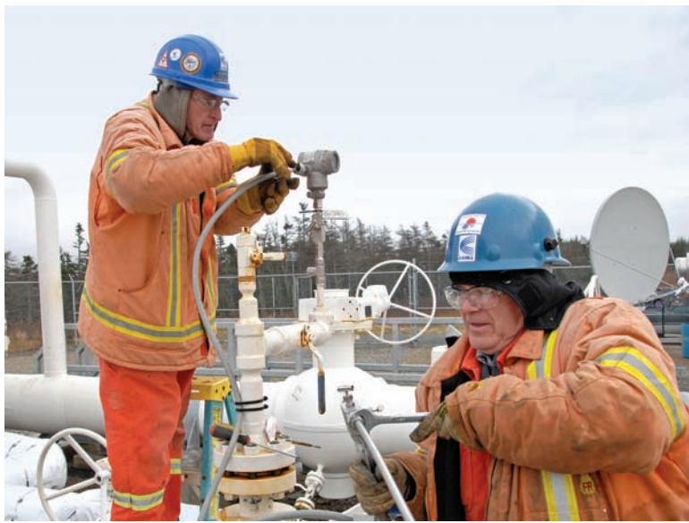
Lyll MacGregor (l), mechanical supervisor with GJ Cahill and Martin Beaver (r), also with GJ Cahill, finalize the hook-up in December 2011 at the Deep Panuke terminus facility at Goldboro, NS.
