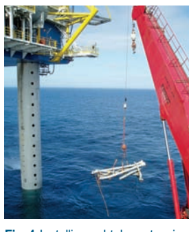
Fig. 4 Installing a J-tube extension frame from Acergy Discovery . At left is the Deep Panuke PFC.
