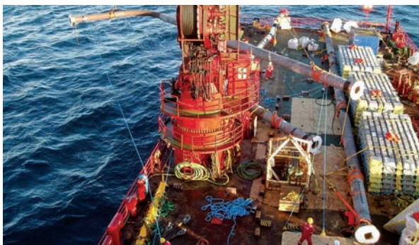
Fig. 3 Overboarding a spool piece for the gas export pipeline from Acergy Discovery to the seabed.
